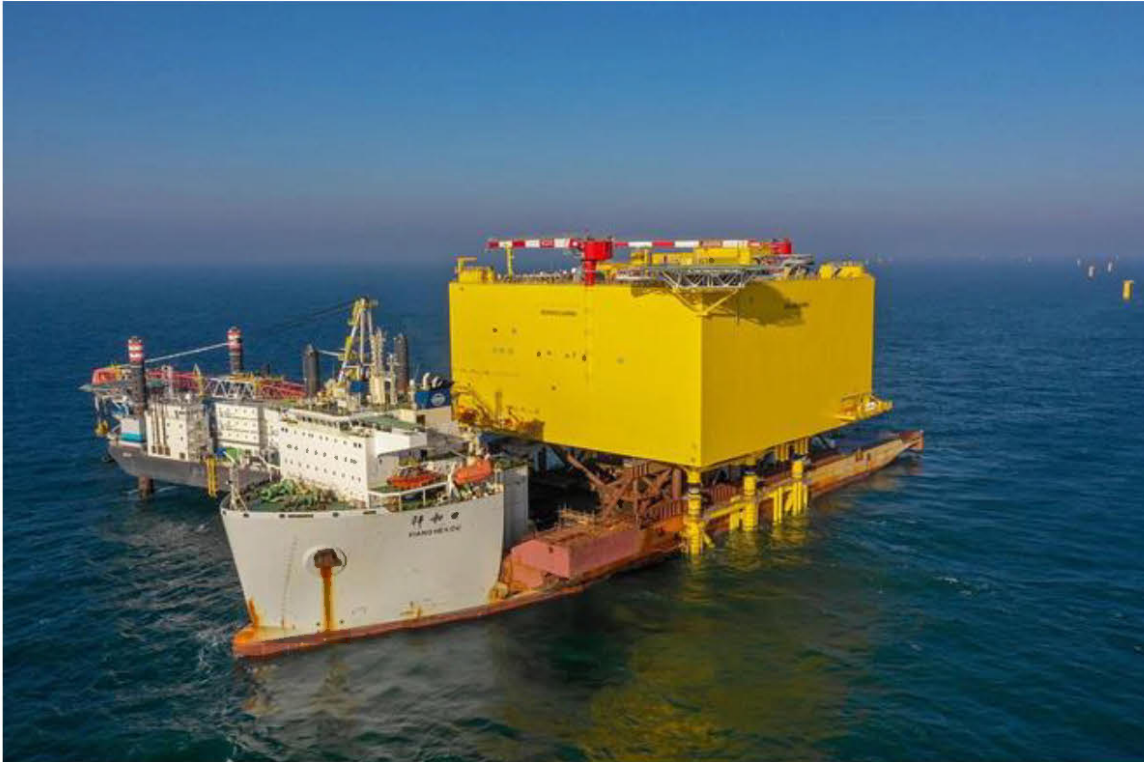
Figure 7b Float over installation of the BorWin3 topside in the German Bight
