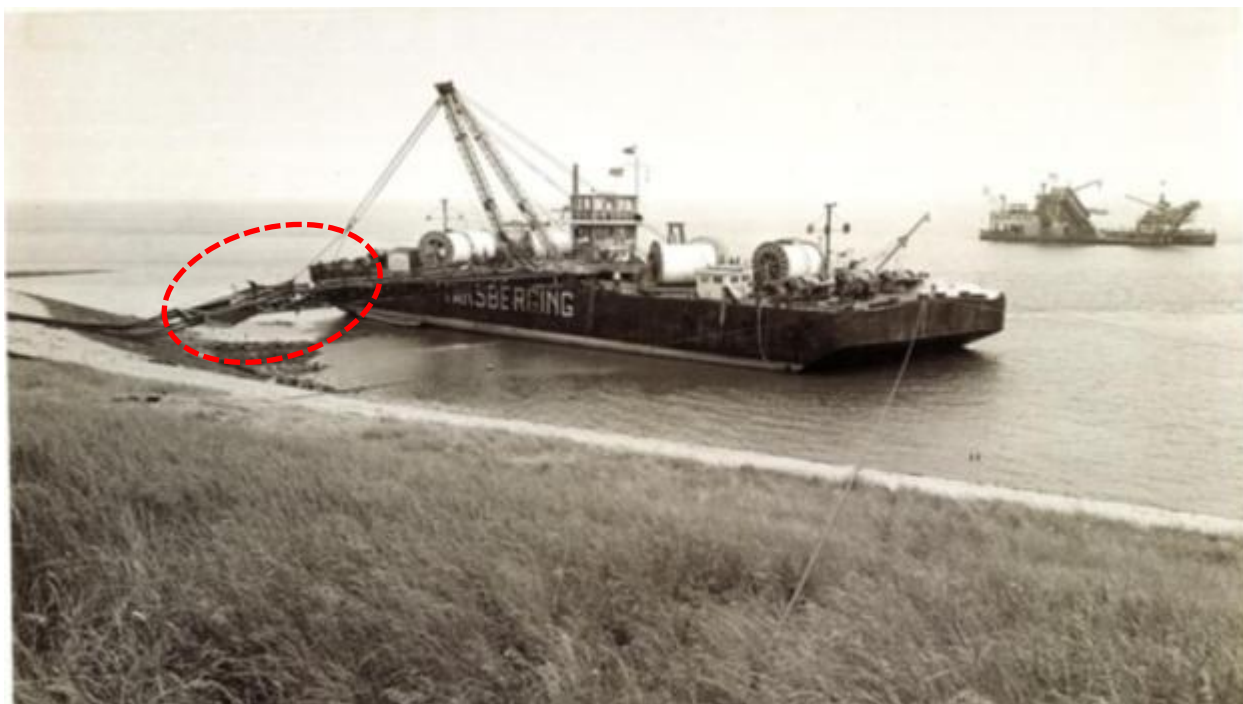
Figure 51 Cable installation by a vertical injector like trencher in Zeeland, location indicated in red
