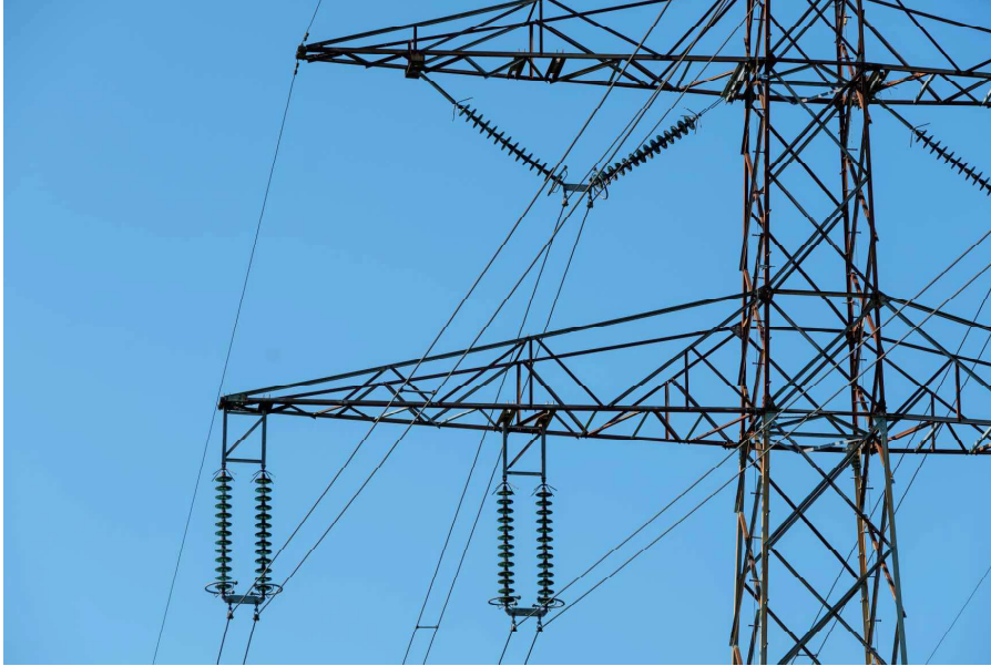
Figure 1 Current suspension phase conductors 150 kV lines between Woensdrecht and Geertruidenberg
