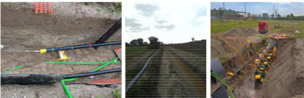
Figure 16 Pull in wire and rollers (left), backfilling before cable pull in (middle), typical roller (right)
