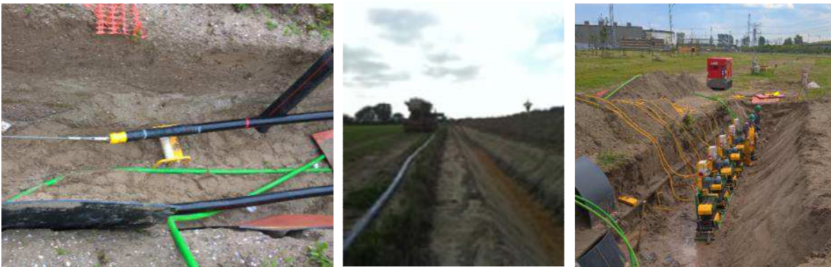
Figure 16 Pull in wire and rollers (left), backfilling before cable pull in (middle), typical roller (right)
