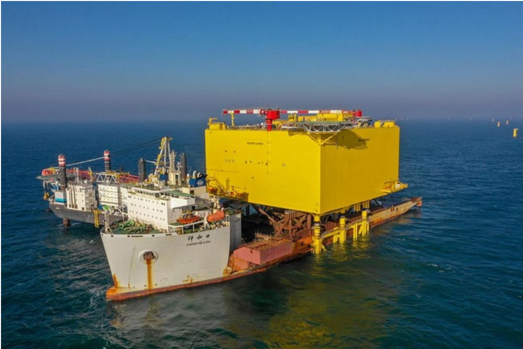
Figure 7a Float over installation of the BorWin3 topside in the German Bight
