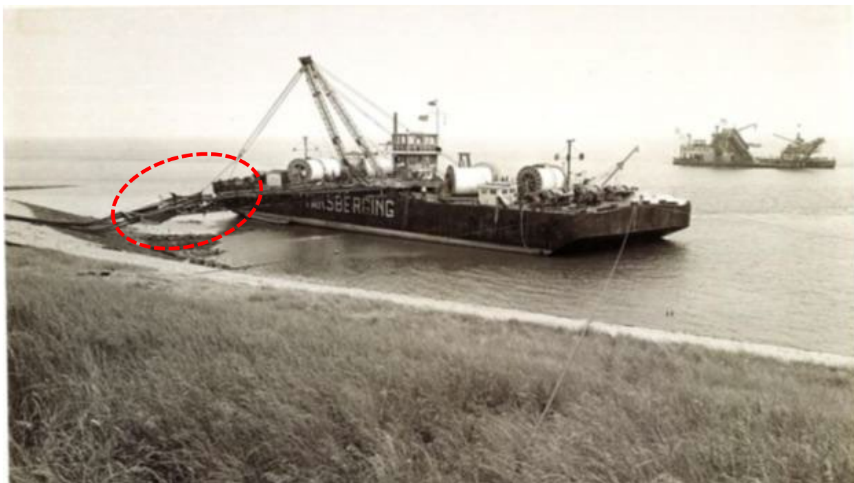
Figure 49 Cable installation by a vertical injector like trencher in Zeeland, location indicated in red
