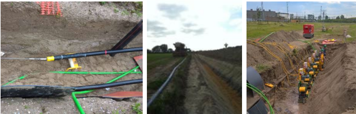
Figure 15 Pull in wire and rollers (left), backfilling before cable pull in (middle), typical roller (right)
