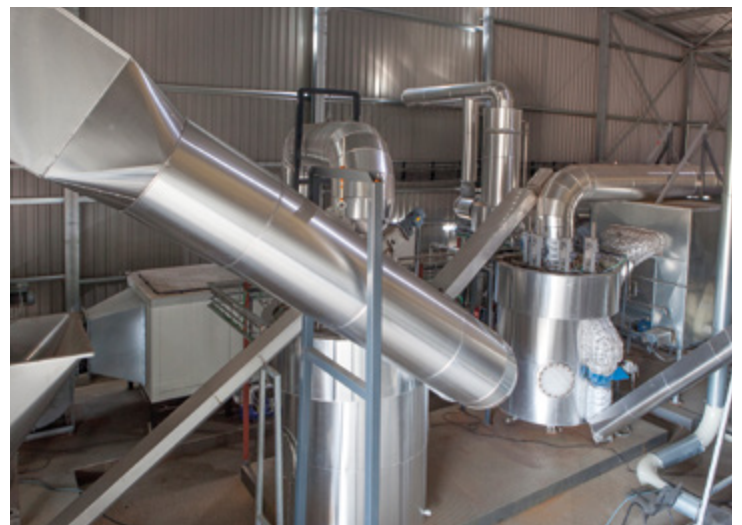
Yilkins' torrefaction technology requires less energy to produce pellets with a high energy value and much lower moisture content. The technology is used by one of the world's largest torrefaction production facilities, in Portugal, which can produce 120,000 tonnes of torrefied pellets and 85,000 tonnes of regular pellets each year.
