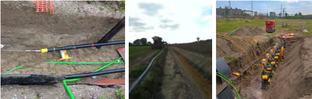
Figure 17 Pull in wire and rollers (left), backfilling before cable pull in (middle), typical roller (right)
