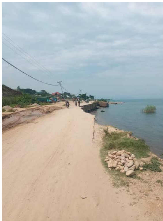
The access road from Uvira is eroding into the lake © Oscar Bahizi
