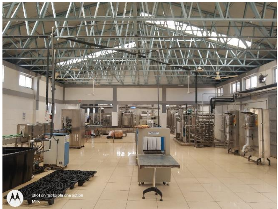
Image 21: Large-scale processing plant, Ekumfi
