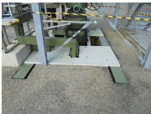
foto 2: Detail installatie / Well Head
