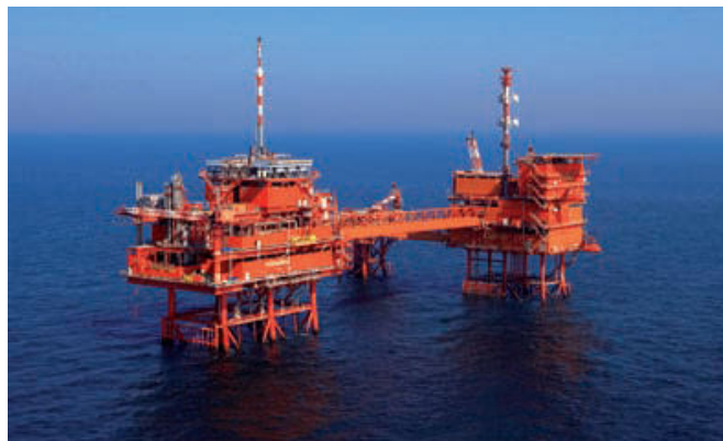
Figure 8.12: P15-ACD Processing & Accommodation Platforms. (Courtesy TAQA; TAQA, 2009)
