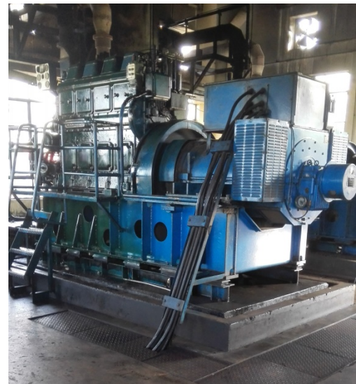
Figure 6: Old diesel generator at Ngara
