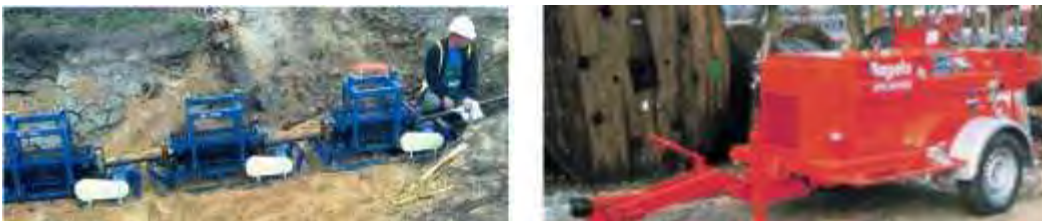
Figure 17 Typical cable tensioners (left) & cable winch (right)
