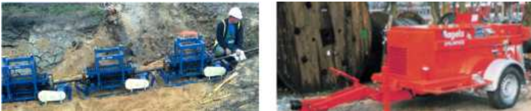
Figure 17 Typical cable tensioners (left) & cable winch (right)
