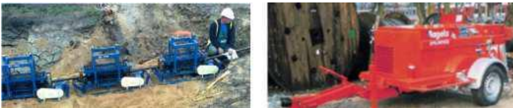
Figure 17 Typical cable tensioners (left) & cable winch (right)
