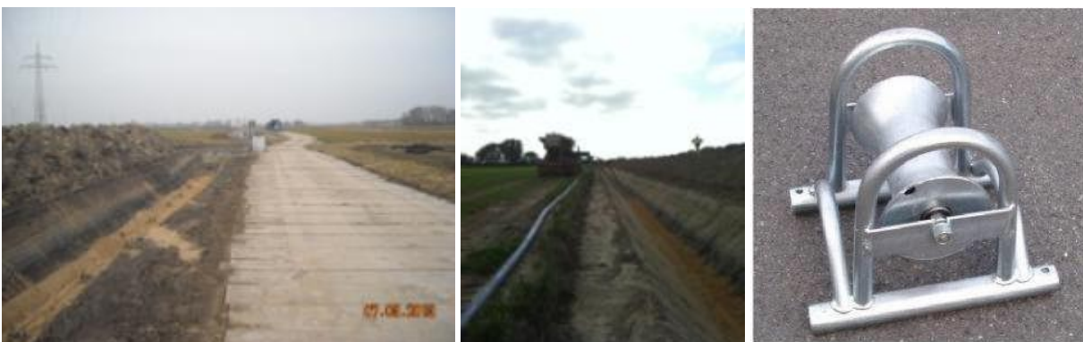
Figure 18 Pull in wire and rollers (left), backfilling before cable pull in (middle), typical roller (right)
