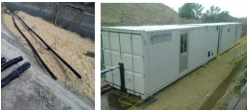
Figure 27 (left) Cable ends in jointing pit – (right) Typical jointing containers
