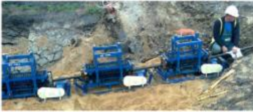
Figure 19 Typical cable tensioners
